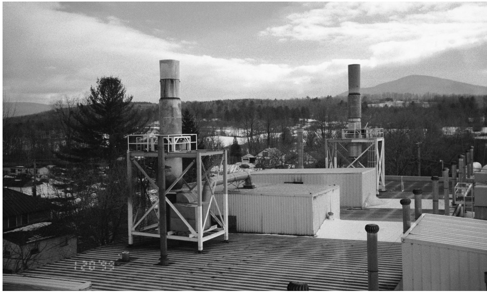
Figure 1. Image from a state inspection of the ChemFab Plastics Factory in Bennington Vermont, January 1999. (Vermont Department of Environmental Conservation)
